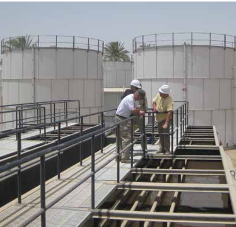
Wastewater Treatment Plant, East End Barracks Housing Complex, Baghdad, Iraq
